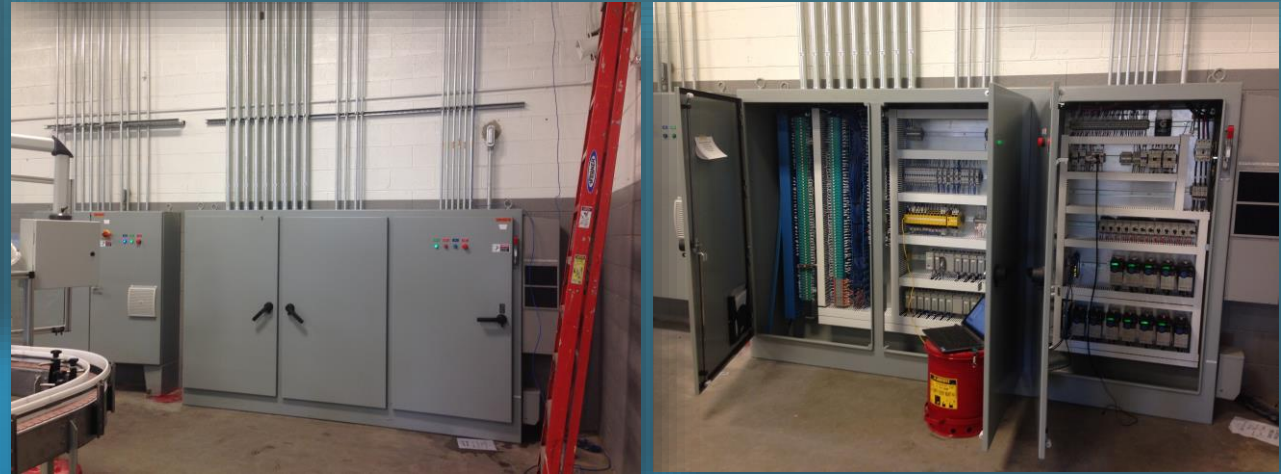
Main electrical panel
