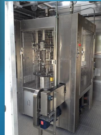
Gassing Machine in Gas House
